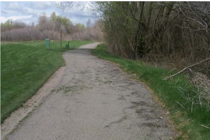
Root Damage to Cart Path #8 Blue Tee
