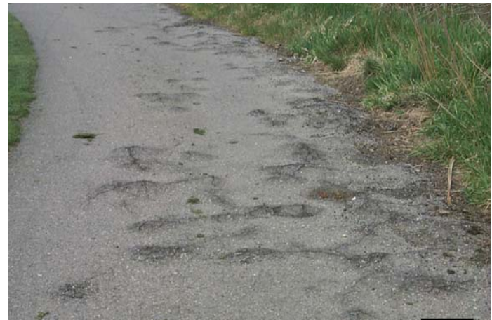
Root Damage to Cart Path #8 Red Tee
